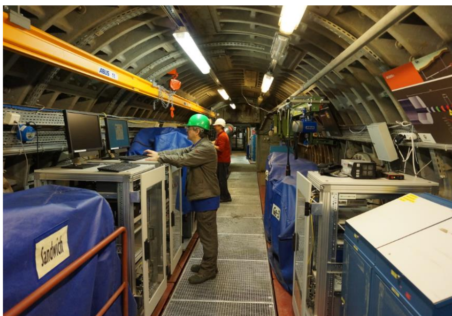
Figure 1. Interior view of the HADES underground research facility showing the area with JRC's HPGe detectors (under blue dust-covers) operated by the RN team of JRC-Geel. Source: JRC with permission from Euridice.
